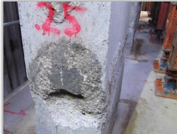
Aggressive/Corrosive ground and groundwater
