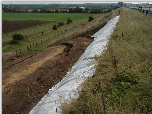
Engineered soil slope failure
