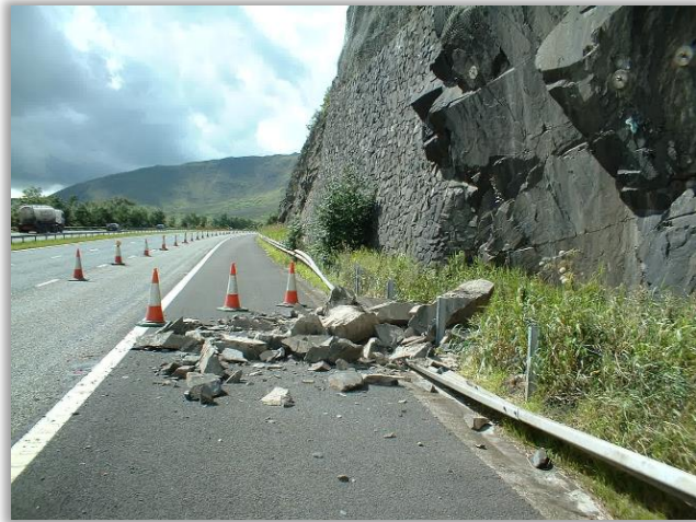
Rock slope failure
